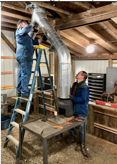
Dan and Jeff install ductwork that vents the coal burning forges we have installed in our blacksmith shop at the Illiana Showgrounds in Rainsville, Indiana. Soon there will be 12 operational forges.
