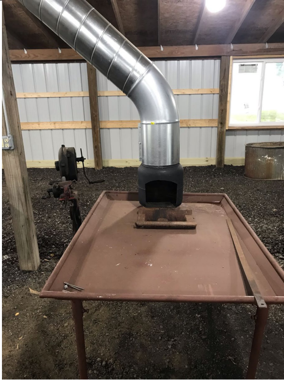
New forge table, fire pot, super-sucker, and vent pipe that exits through the roof.
