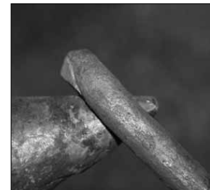
Fig. 6. Move to the tip of the horn, hold the link at 45° and continue to weld
